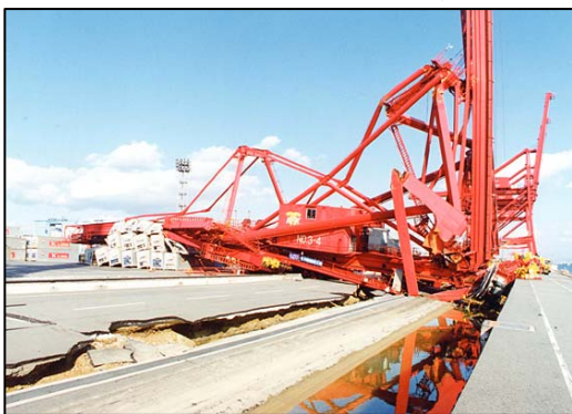
Figure 3 Earthquake-induced port damage
